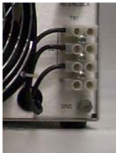
Figure 5-3. AC Power Connections.
